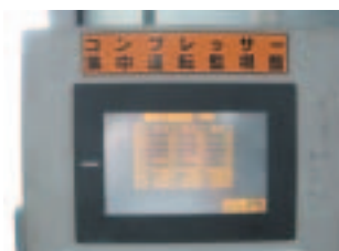
■A monitor display showing the volume of compressed-air flows
