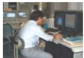
Central monitoring room
